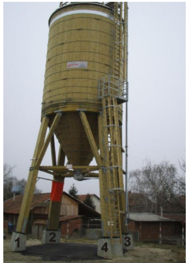
Figure 4. Salt silo: a) Silo photograph b) Silo foundations at the depth of 1.3 m, diagram of the foundations and driven-in micro-piles
