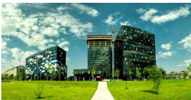
Figure 1. A view on the smaller tower which is finished and on bigger under construction
