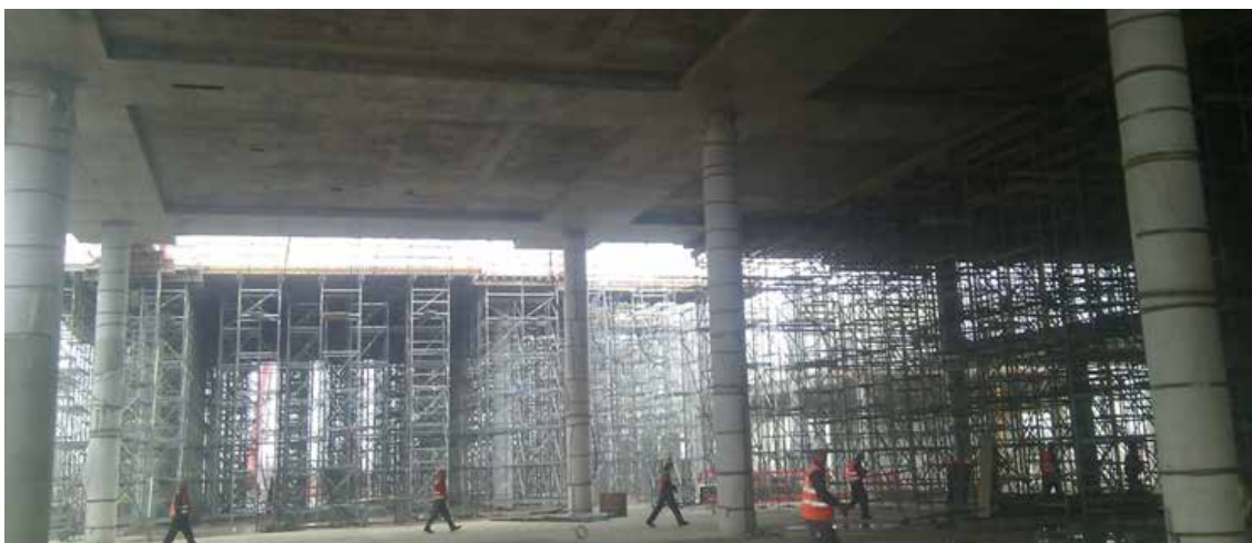
Figure 9. A view on the first floor slab with span 14.4x14.4 m, middle zone, columns height 10 meters through two levels
